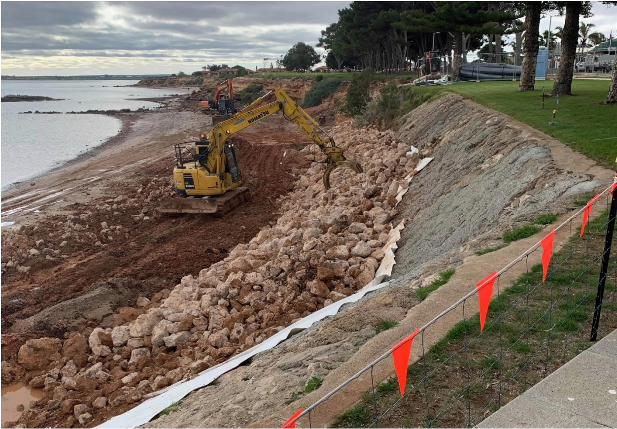
Council undertook revetment works on the Ceduna Foreshore during 2020. Hard Revetment wall works are planned for Smoky Bay Foreshore with assistance from Coastal Protection grant funding.
